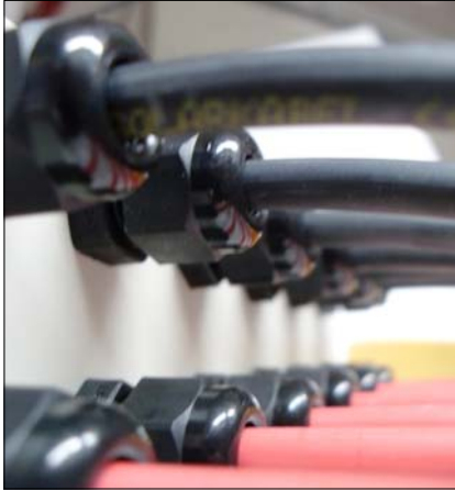
Figure 7: Output Electrical Leads
